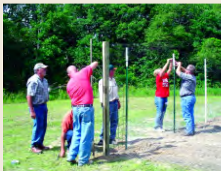
Workers and volunteers installed an eight-foot fence around plots of biopharmaceutical corn planted at the Iowa Army Ammunition Plant near Middletown.
